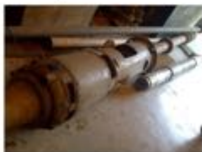
Pump Service – Pembangkit Jawa Bali UP. Muara Karang
